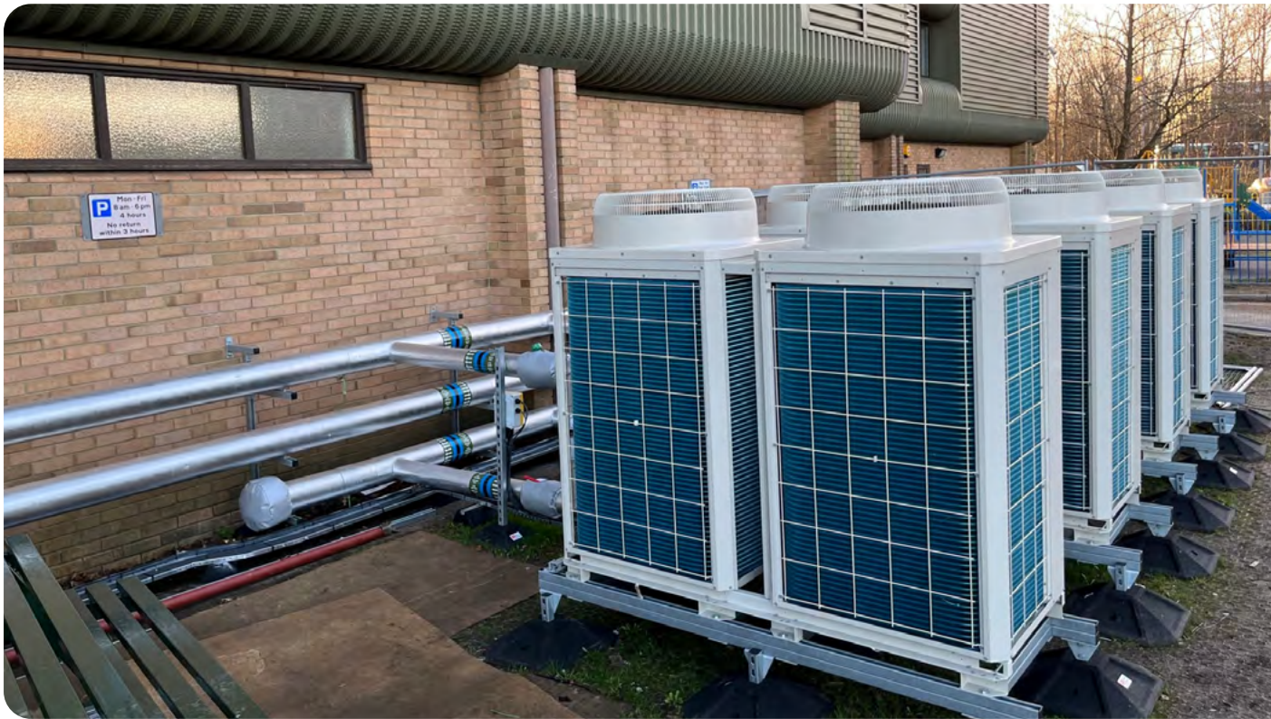
Heat pumps providing heat to Abbey Leisure Centre
