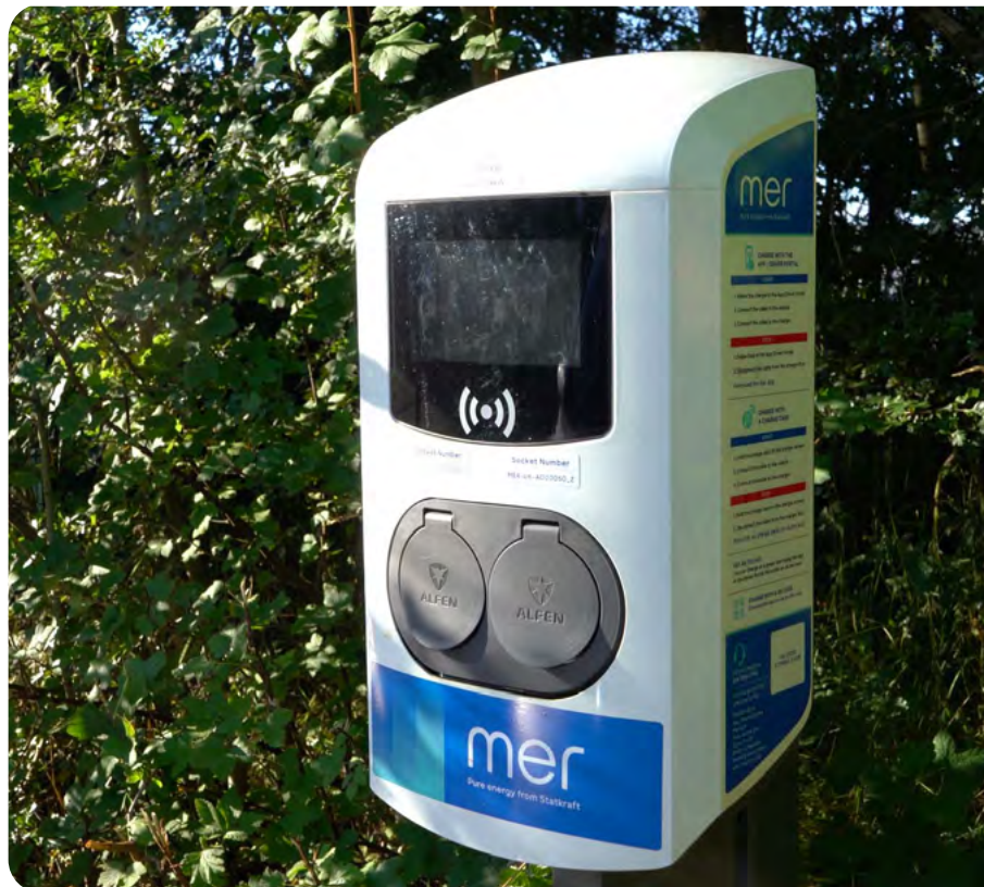
Electric vehicle charging point.
