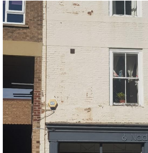
Fig 4, image of general fabric issues collapsed historic wall, render issues, and joinery decay.
