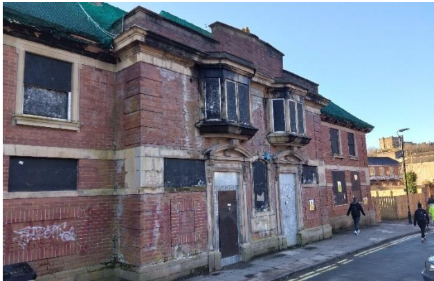
Fig 3, above, example of a two long term disused and deteriorated historic building, the former public swimming baths a historic landmark building on the riverside.
