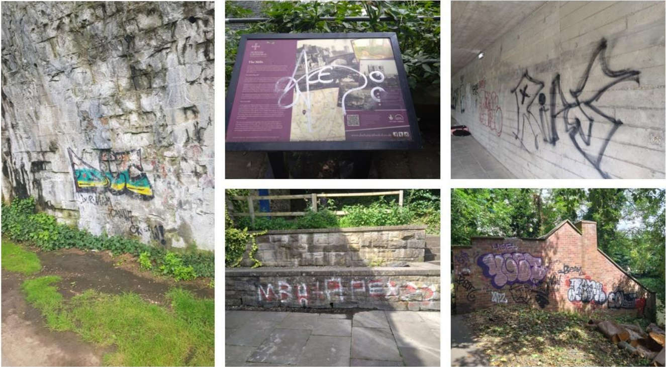
Fig 57 different examples of graffiti that harm the fabric and visual appearance of the historic environment.
