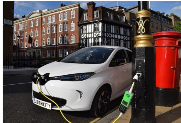
Fig 67 above, examples of a free standing at Sidegate carpark and a lamppost electric vehicle charging point product in London.
