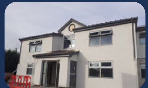
A building being retrofitted with insulation as part of the low carbon depot project.
