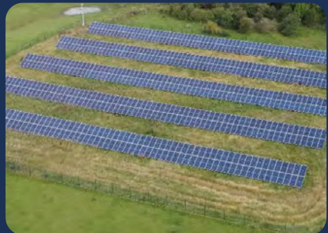
Tanfield Lea Solar Farm. A 250kW solar farm providing green electricity to a Durham County Council office building.
