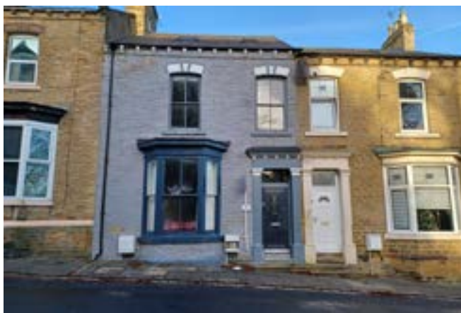
Painted stonework is both damaging to the building’s fabric but also disrupts the appearance of an otherwise uniform terrace
