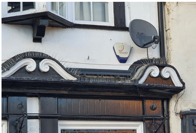
Bird spikes and the satellite dish are visually intrusive
