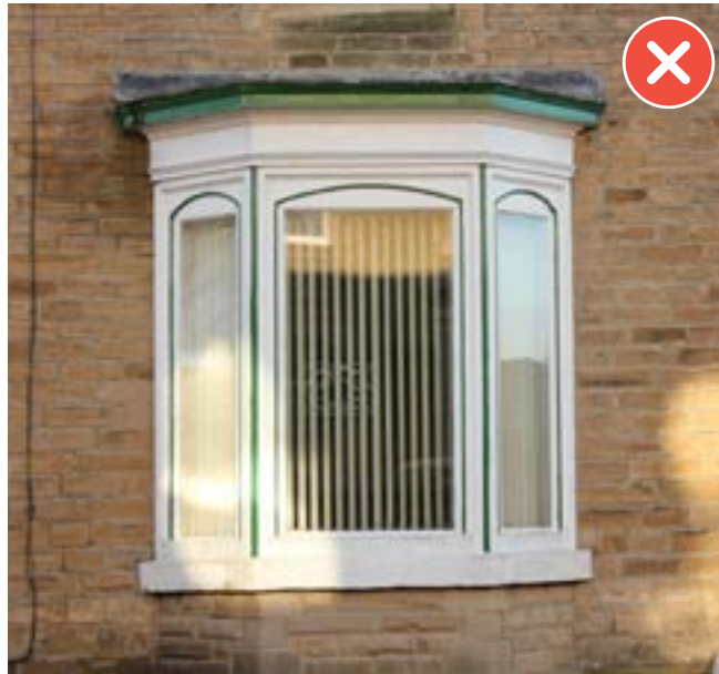
Inappropriately designed window insert into a historic bay window
