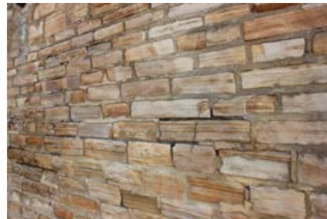
Poorly pointed stone wall
