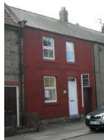
Loss of historic detailing, properties on Winston Road
