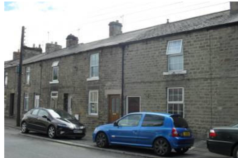
Loss of historic detailing, properties on Winston Road
