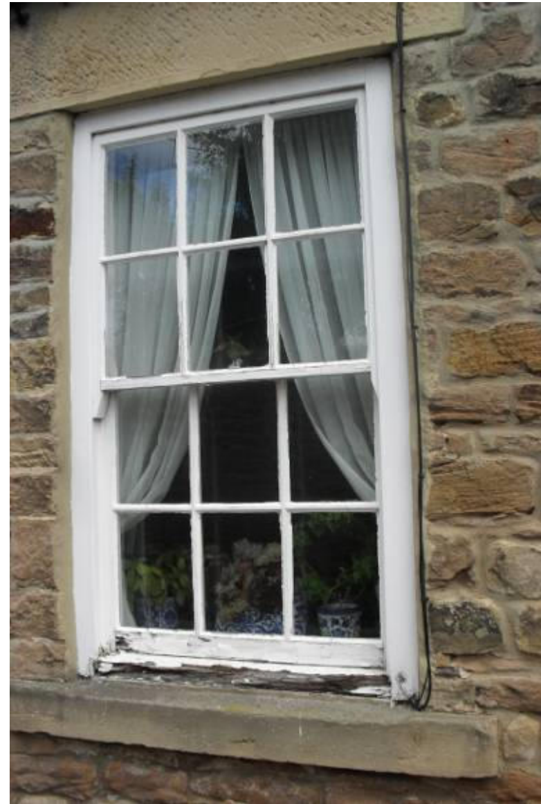
Sash window in poor condition
