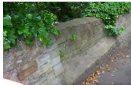
Seat built into the wall on Church Bank – in need of repair
