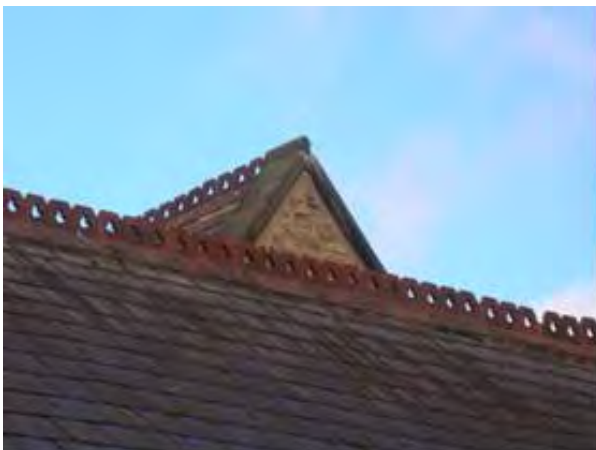
Terracotta ridge tiles have been used to add interest to the slate roof of the Methodist church
