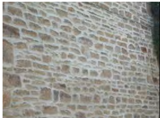
Good quality lime mortar pointing that respects the stone and allows it to breath
