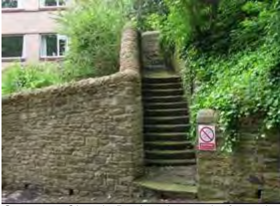
Steps on Church Bank – in need of repair and restoration
