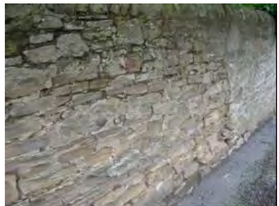
Stone boundary wall that has been maintained inappropriately with cement pointing, hastening the rate of erosion.
