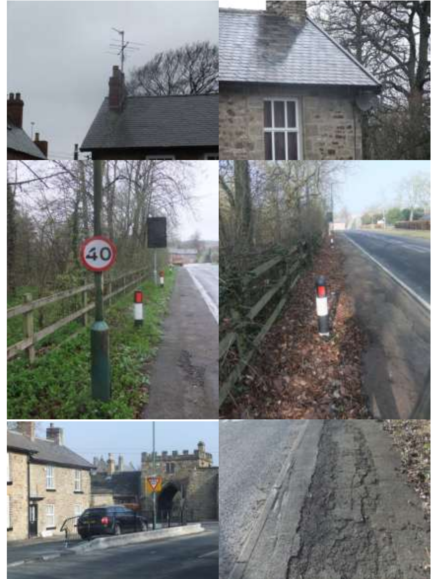
Examples of prominent TV aerials and satellite dish, road side clutter and poor surfaces.
