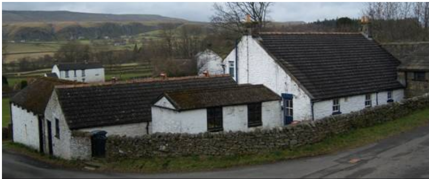
A variety of roofs including stone flags, tiles, artificial slates with red ridge tiles and corrugated sheeting at Pleasant View
