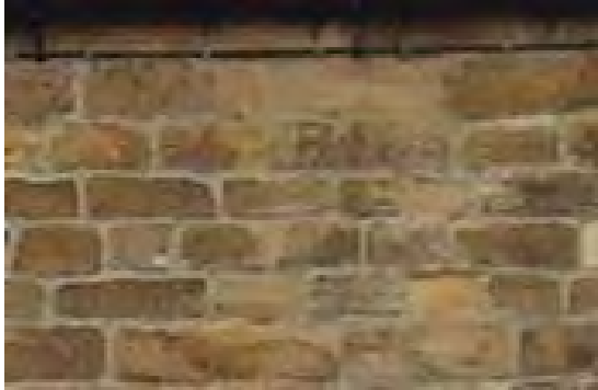
Squared coursed stone is often used for front elevations and rubble construction for the side and rear
