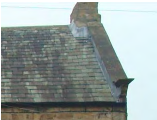
A graduated Lakeland slate roof with stone waterboard and kneelers – typical of the buildings in the core of the village.
