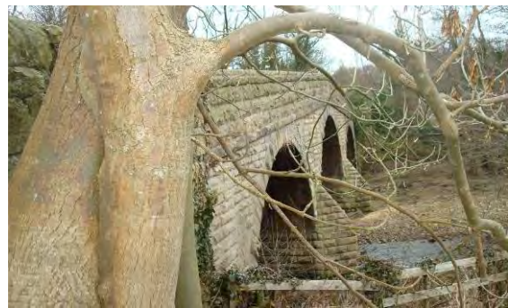
Ebchester Bridge – this was once the main crossing of the River Derwent, but is now only a footbridge
