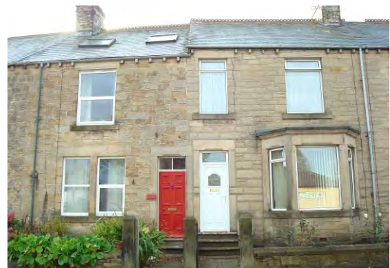
Many of the traditional door and window details have been lost. No. 4 has a traditional door, which is part of the design of the building and contributes to its interest
