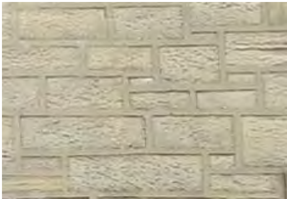
An example of inappropriate cement pointing that stands proud of the stone
