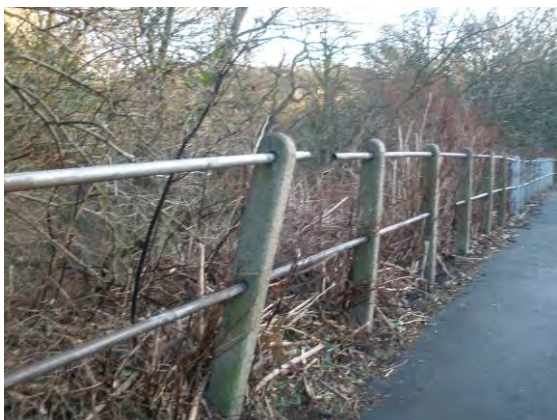
Barriers between the roads and woodland – some are in need of repair
