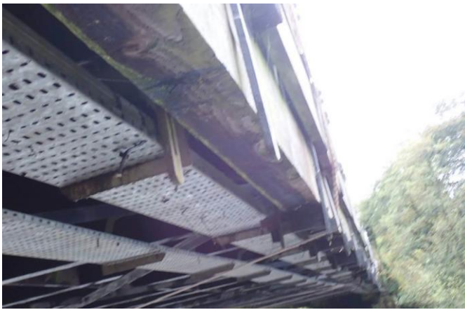
Image 5 - Missing securing wedges
