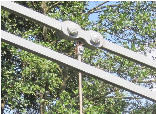
Image 2 - Broken hanger to west elevation
