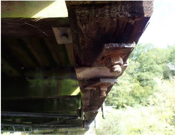
Image 1 - Typical condition of longitudinal timber and loose bolts
