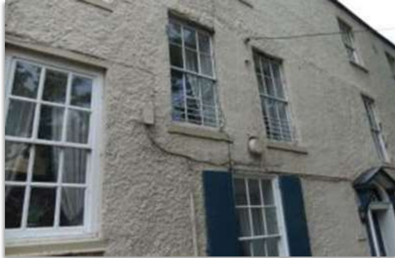
Image 27 A cluttered elevation with prominent alarm box, service box and wiring
