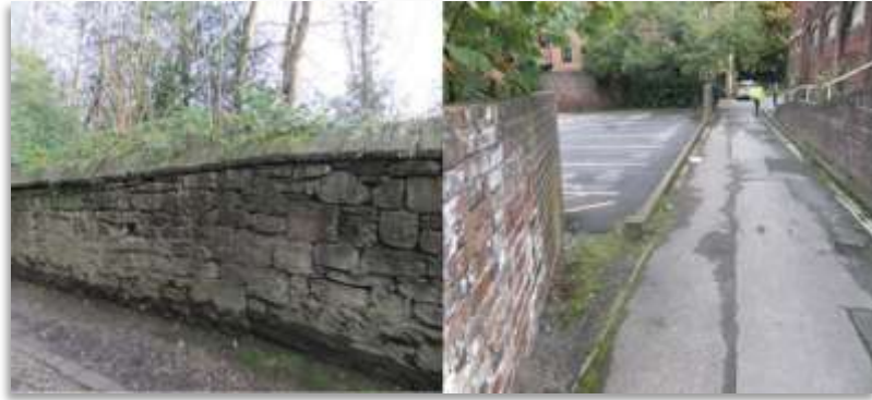
Image 29 Example of erosion to historic stone wall and loss of part of brick boundary wall
