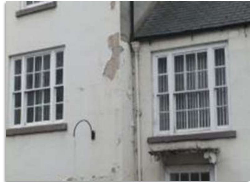
Image 25 Example of a lack of building maintenance
