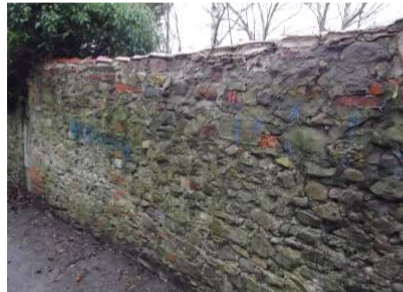
Image 22 Issues with maintenance and graffiti
